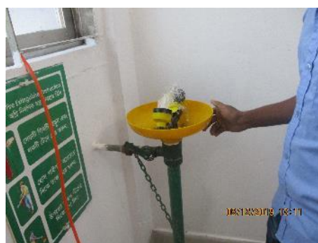
Eye Wash Station
